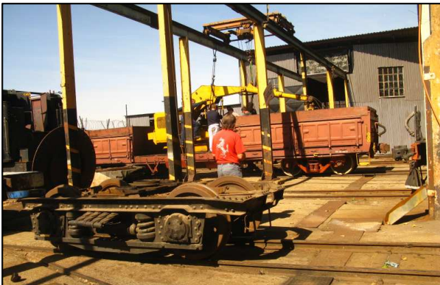
P03 - Engineering Apprentices being guided on removing the hydraulic rams from the Coal Grab. In the foreground is the Locomotion Bogie after bolster hardware cleaning.
