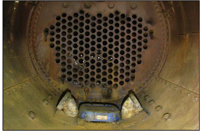
P04 - Class 6A 473 Charlotte's simple front tube plate after having had all the boiler tubes removed.
